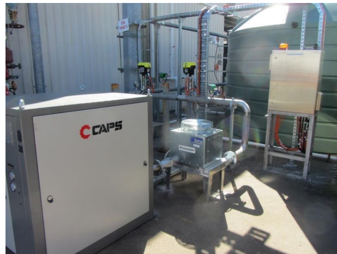
Photo 1: Blower, cooler, control cabinet and piping.
